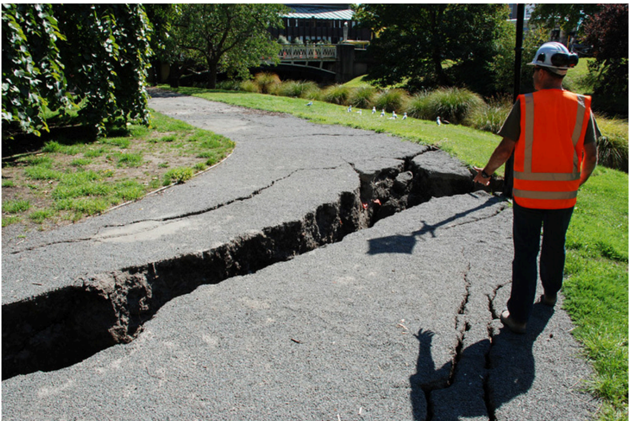
Image 3: Damage caused by the 2011 Christchurch earthquake.
